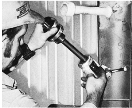
Reseating tool is lowered into valve body after removal of yoke bushing and valve stem.
